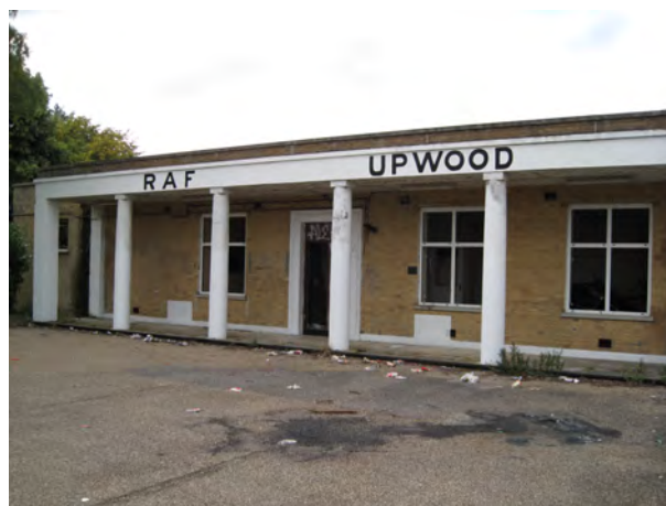
RAF Upwood contains a wide range of former military buildings, mostly of utilitarian architecture, vandalism and decay are damaging the historic character of the site
